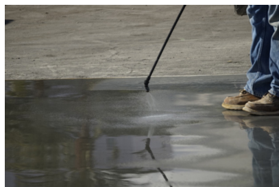
Applying SlabArmor Closer to complete the job. SlabArmor treatment is up to a depth of >25mm (>0.98").
